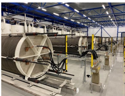
Fig. 9. The 20 MW alkaline electrolyzer plant, which provides hydrogen to the operations at Ovako Hofors.
