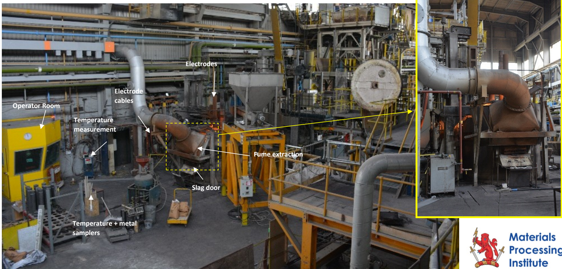
Electric Arc Furnace Setup at Normanton Pilot Plant, MPI
